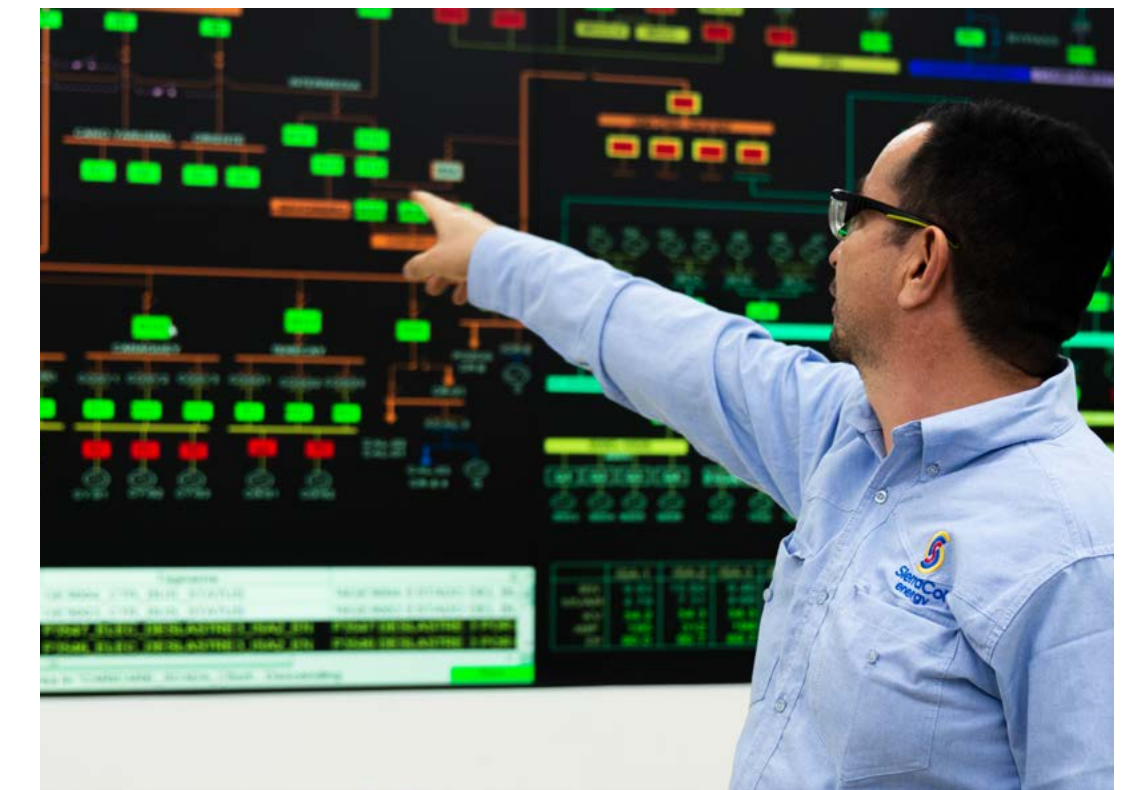
Control room, Caño Limón area
