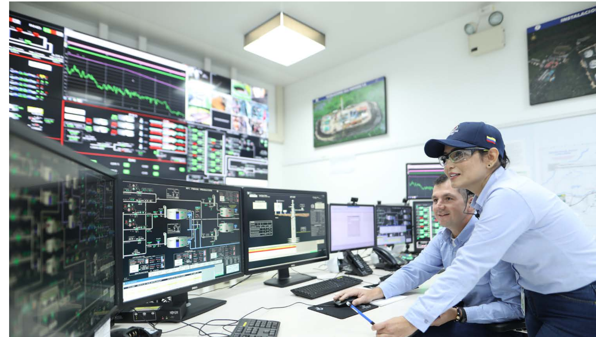
Control room, Caño Limón area
