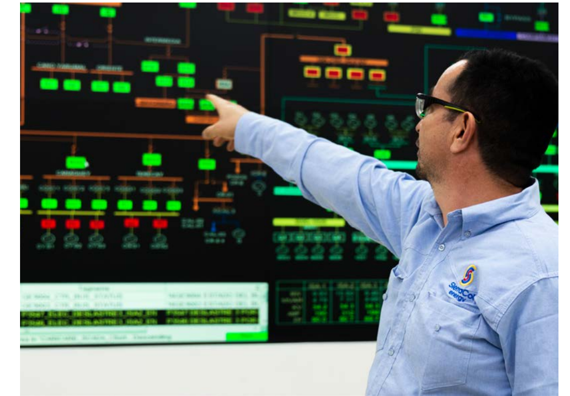
Control room, Caño Limón area
