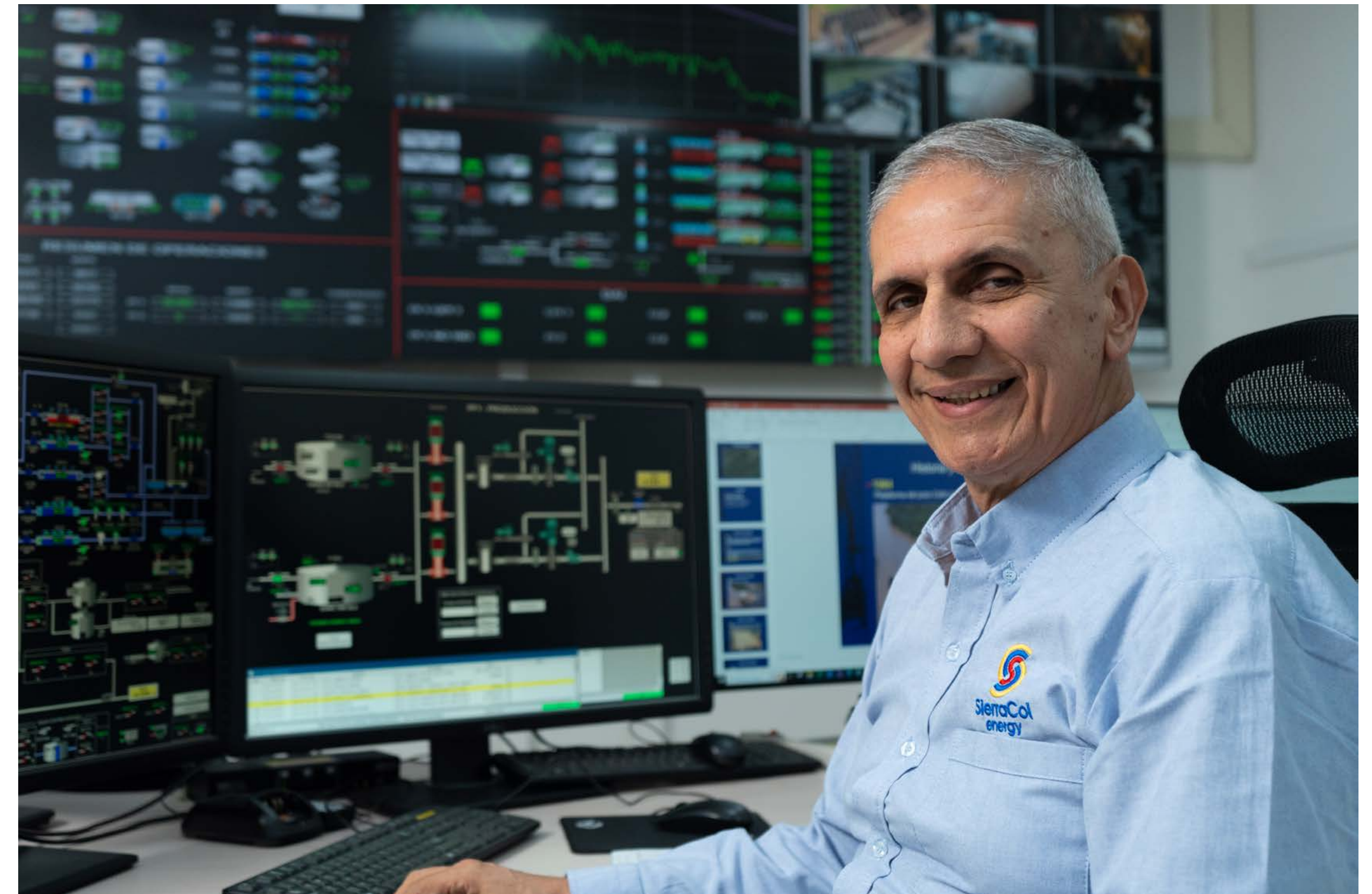
Control room, Caño Limón area
